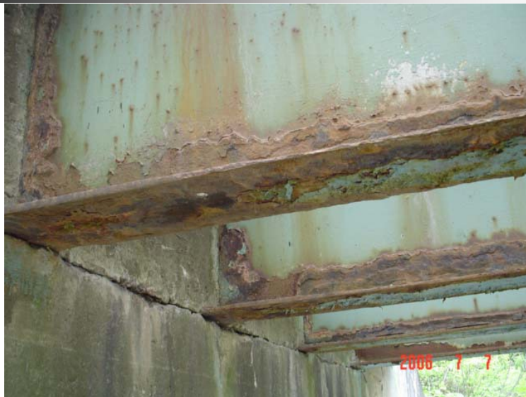
Bottom flange section loss and rusting of webs near backwall in Somerset County (SR 2037)
