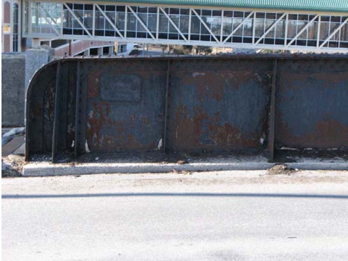
Web deterioration on SR 743 in Hershey – January 2008
